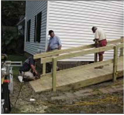
MMIA makes returning soldiers' home safe and workable with repairs and additions such as wheelchair ramps.
